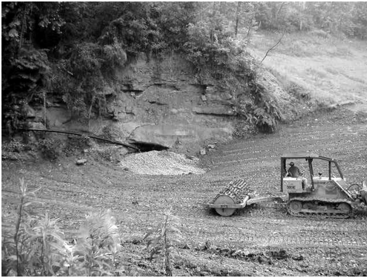
Perry Reclaiming workers filled the Congo Run subsidence hole with 155 tons of stone this June. Photo: Cara Hardesty.
