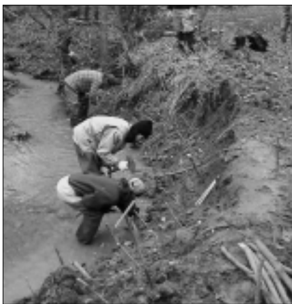
Karyn Tremper and Robin Bowman plant willow posts on an eroded stream bank in Indian Run, Perry County.
