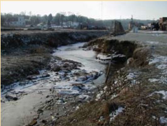
Lack of Riparian Buffer increases stream bank erosion
